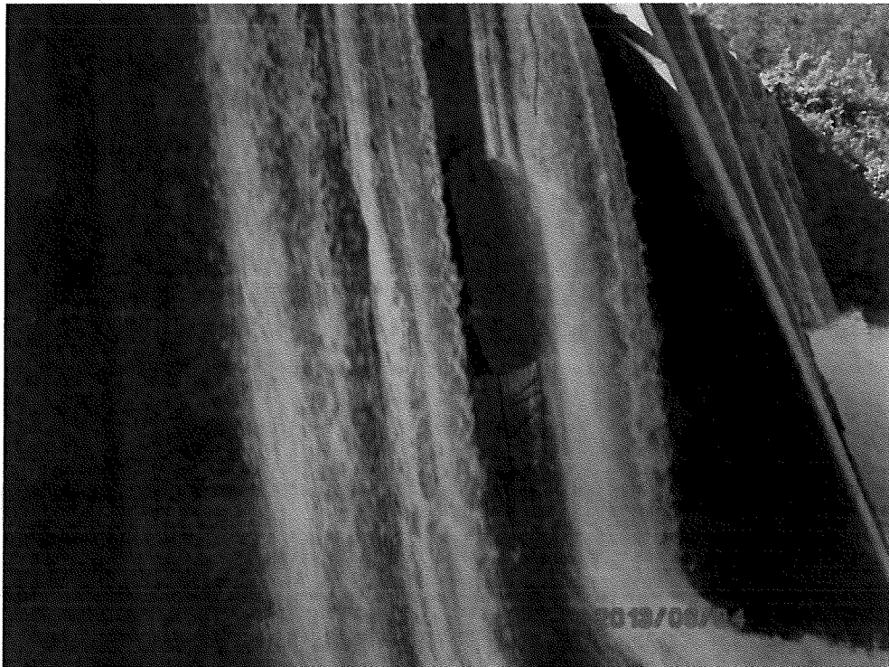
Photo 83 – Spalling concrete on spillway.
