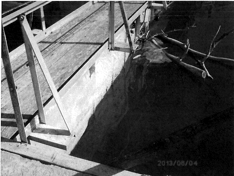
Photo 82 – Exposed concrete reinforcement on reservoir side of McGowan Dam.
