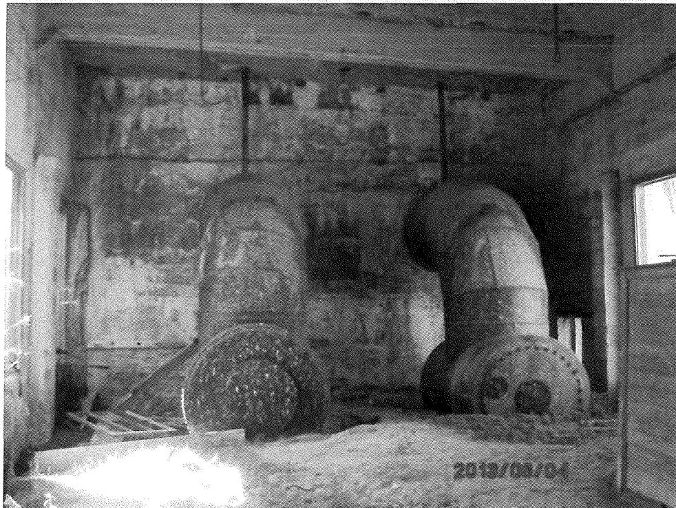
Photo 68 – Penstocks inside powerhouse.
