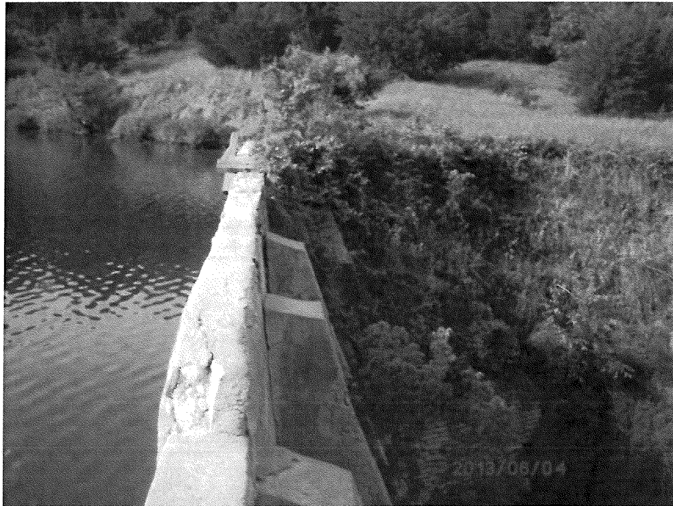
Photo 81- Separation between buttress wall and downstream dam face.
